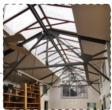
EXISTING TRUSSES TO BE RE-USED, ANY NEW TO MATCH EXISTING AS NECESSARY
