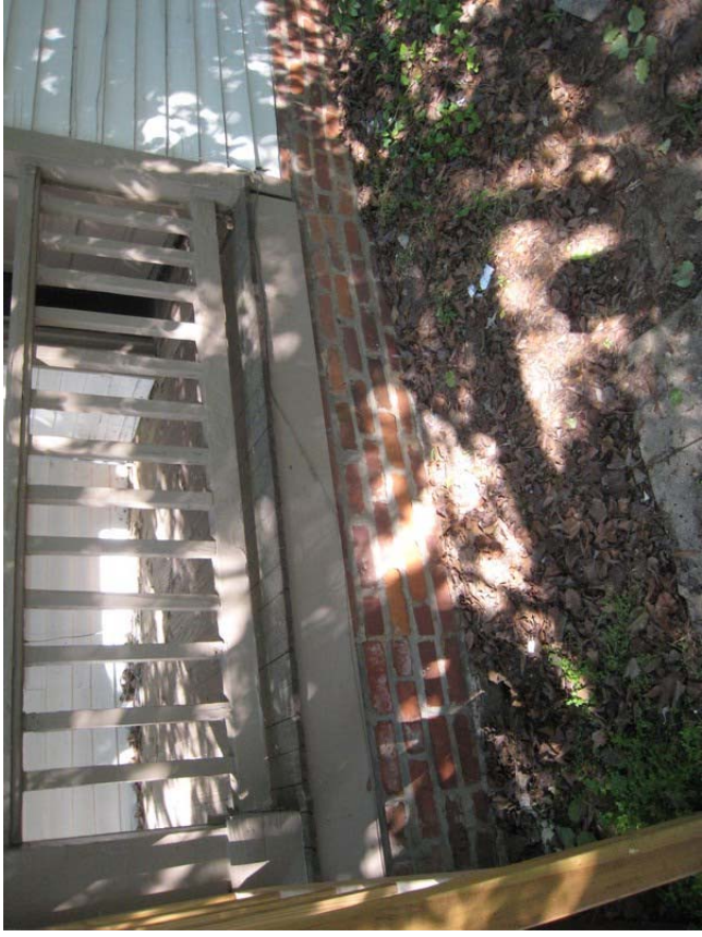
Brick infill reveals original location of steps at end of front walk
