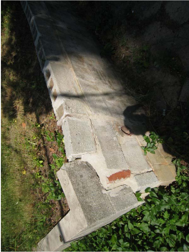
Dilapidated front retaining wall to be replaced
