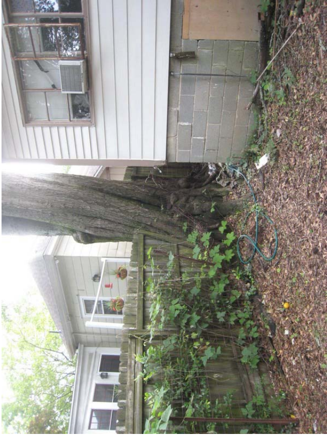
CMU foundation to be repaired after removal of tree and coated with stucco parge coat
