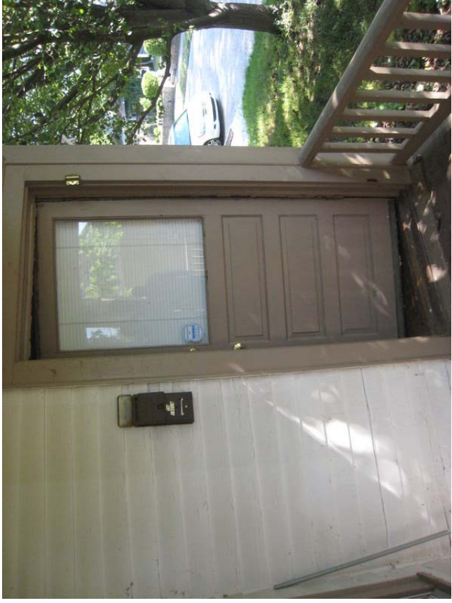
Non-original Unit B (right side) door to be removed
