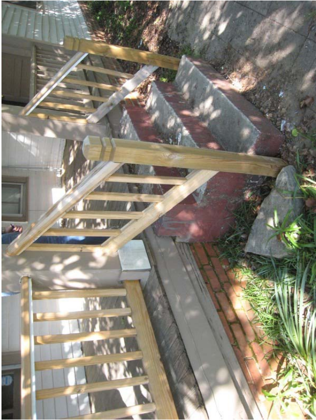
Non-historic porch columns, rails, and steps to be replaced
