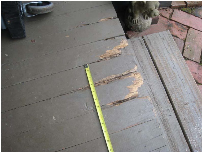
Rotten front porch boards to be replaced in-kind
